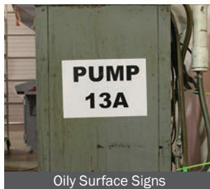
Oily Surface Signs
