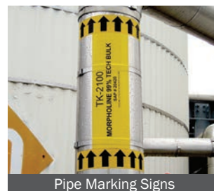
Pipe Marking Signs
